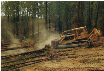
Firebreak being constructed outside of Kelowna (2003). Photograph by Gary Nylander, from Firestorm .
