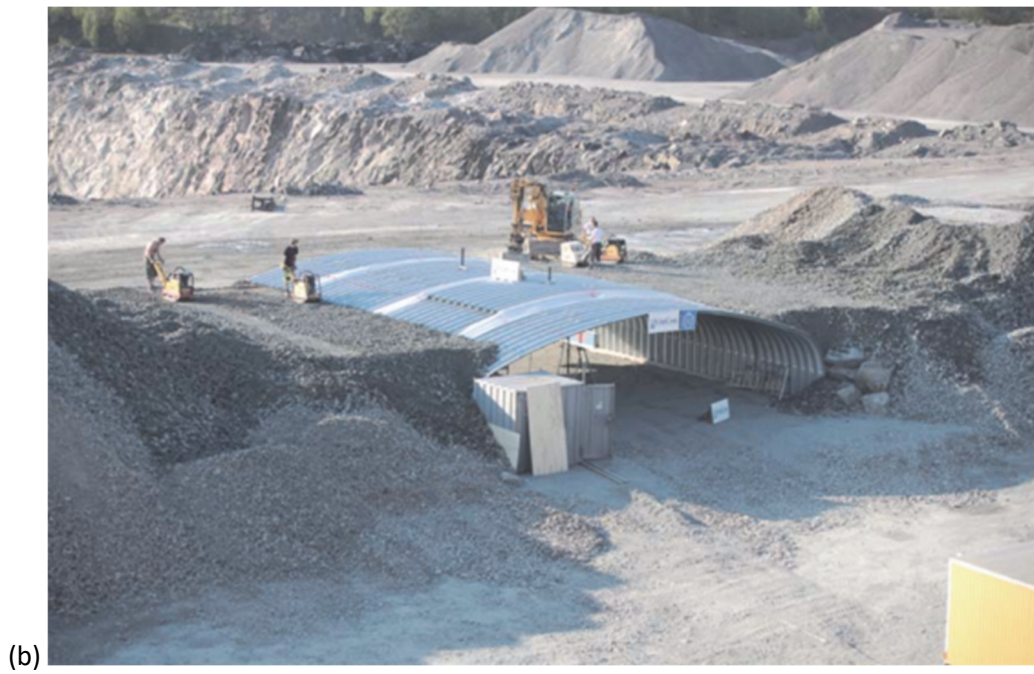
Figure 3.2. (a) Assembling of the box culverts and (b) compaction of the backfill
