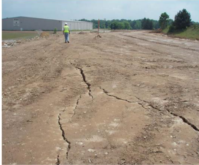
Figure 2.18: Tension cracks appeared on top of the embankment at site (Timothy 2017)
