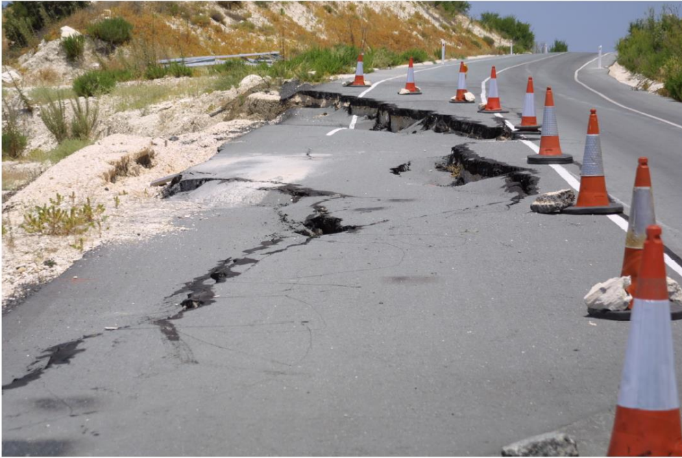
Figure 2.11: Cracks developed at the Pentalia road in July 2005 (Hadjigeorgiou 2012)
