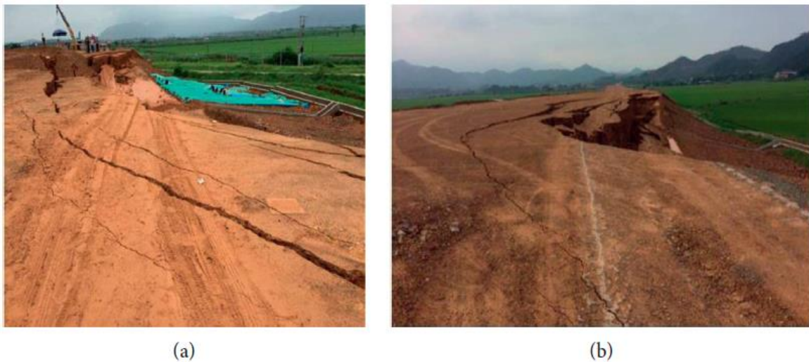
Figure 2.12: Sliding observed towards (a) The left of the embankment (b) The right of the embankment (Shaofu 2020)
