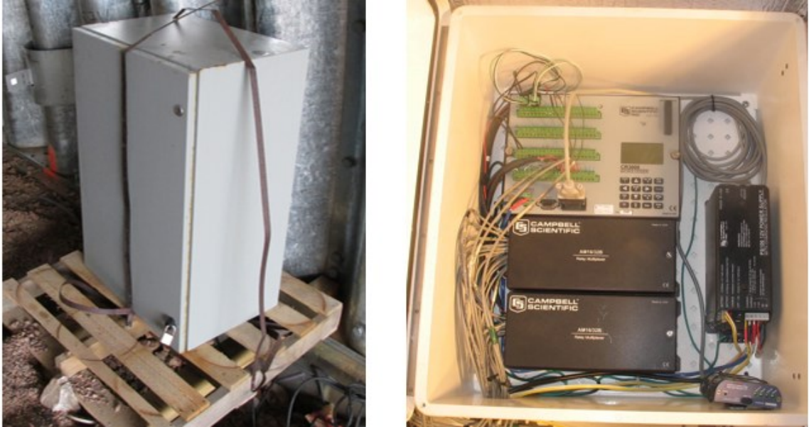
Figure 4-14: a) Steel box b) data Logger and components in plastic enclosure
