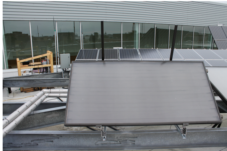
Figure 4.4: Top: Ground location (shaded), bottom: Roof location (unshaded)
