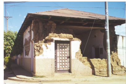
Adobe house showing damage after an earthquake (Lopez et al. 2004)
