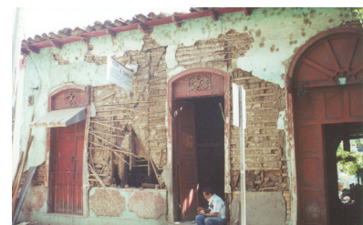
Bahareque dwelling in San Vicente showing damage after an earthquake (Lang et al. 2007)
