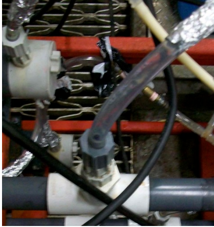
Figure 3.6 Influent port for the pipe loop
