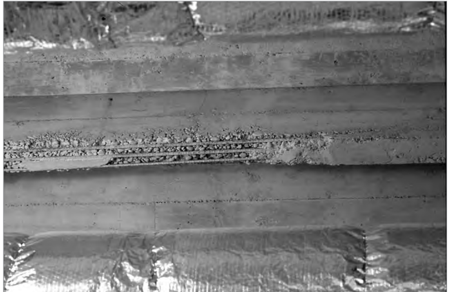
FIG. 3. DETAIL OF EXPOSE REBAR IN WALLING LOCATED INSIDE THE SPIRE. ST. PATRICK'S ROMAN CATHOLIC CHURCH, MEDICINE HAT, ALTA. (1912-1914). | BARRY MAGRILL.
