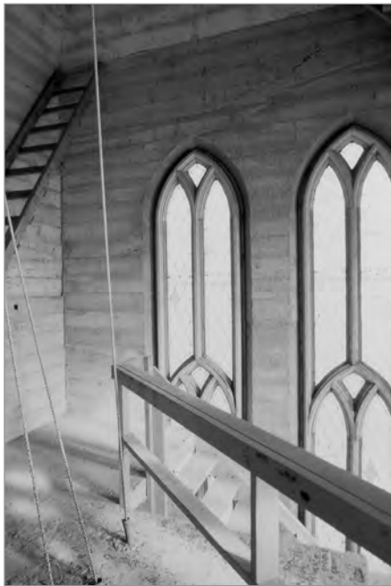
FIG. 2. DETAIL OF THE INTERIOR OF THE CHURCH TOWER REVEALING THE FORMWORK IMPRINTS LEFT BEHIND AS THE METHOD OF CONSTRUCTION. ST. PATRICK'S ROMAN CATHOLIC CHURCH, MEDICINE HAT, ALTA. (1912-1914). | BARRY MAGRILL.
