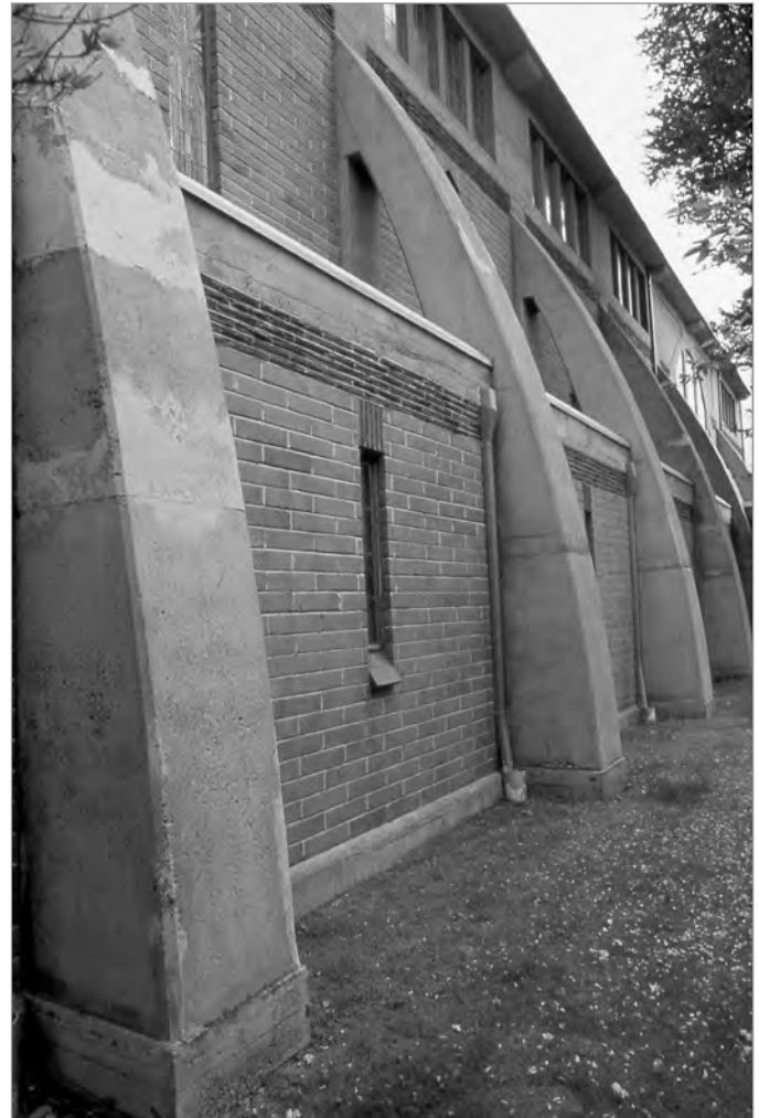
FIG. 8. DETAIL OF BUTTRESS, VIEW OF THE SOUTH SIDE OF ST. JOHN'S ANGLICAN CHURCH, SHAUGHNESSY, VANCOUVER, B.C. (1949), SHOWING THE TRAJECTORY OF THE REINFORCED CONCRETE BUTTRESSES. | BARRY MAGRILL.
