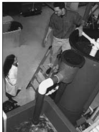
A recirculation system with its biofilter system.
