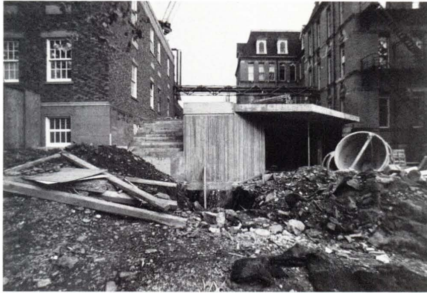
New entrance into the dental building located between the Forrest Building and the "old" dental building takes shape
