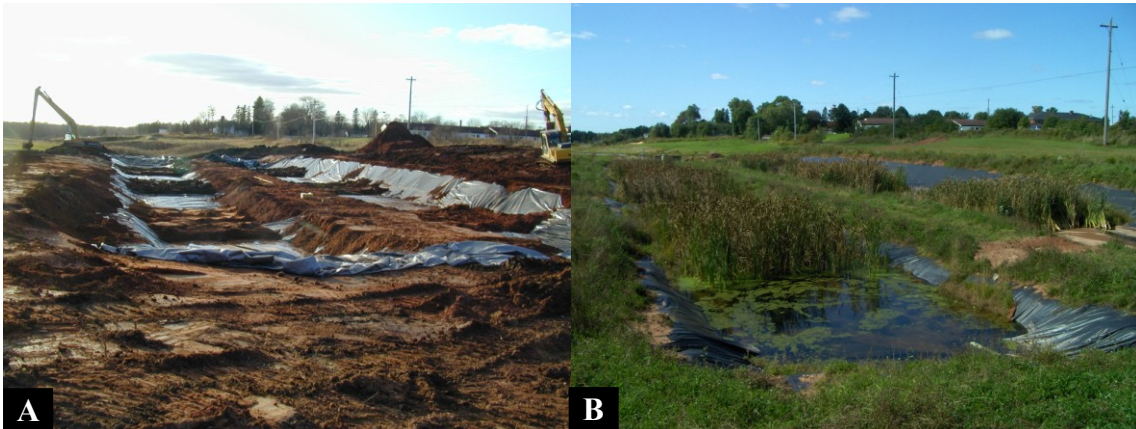
Figure 3.5 (A) Constructed treatment wetlands during construction in November 2006 and (B) in September 2008.
