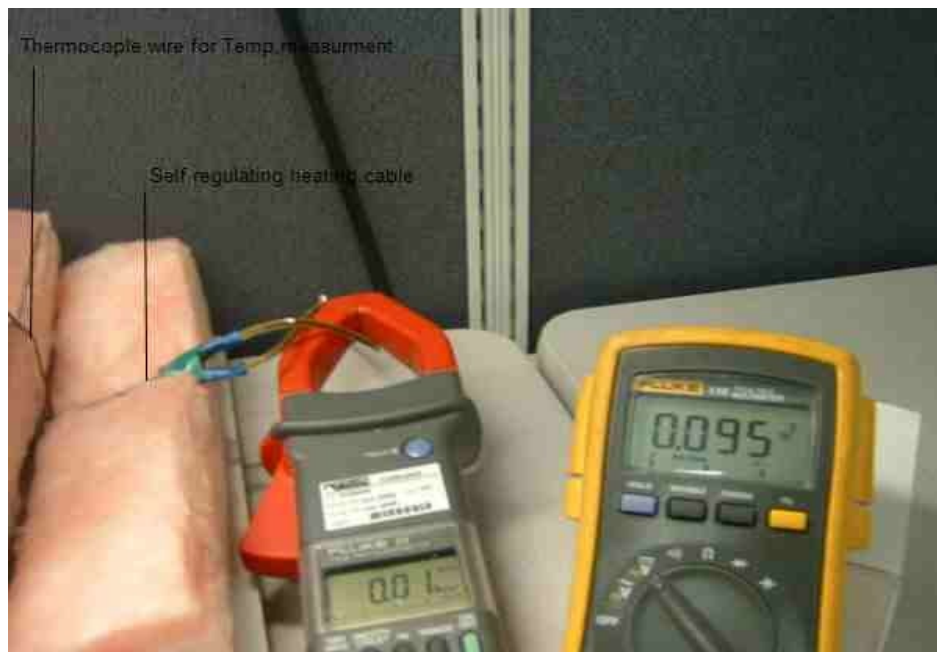
Figure 5.26: Stage-2 Maximum temp. of self-regulating cable observed at 10.40AM.
