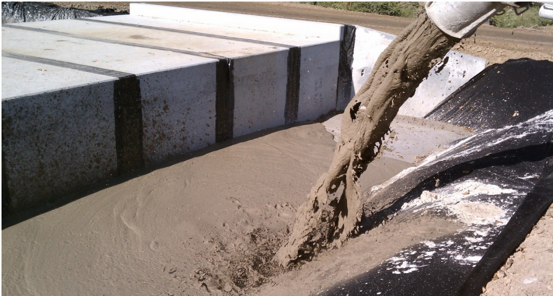
Figure 2-6: Use of CLSM to fill the backfill in a project. Source: ( https://ohioreadymix.com/ )
