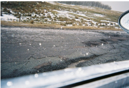
Figure 7 James' photo 1 of potholes.
