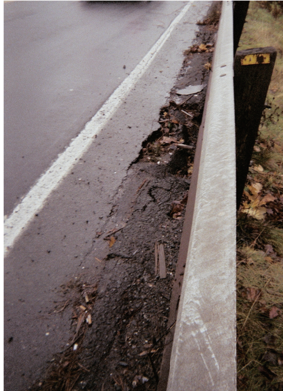
Figure 3. Cracked pavement on the shoulder of the road.
