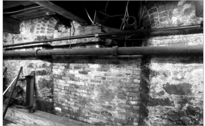
FIG. 8. PARIS TOWN HALL, INTERIOR, BLOCKED E DOORWAY. | MALCOLM THURLBY
