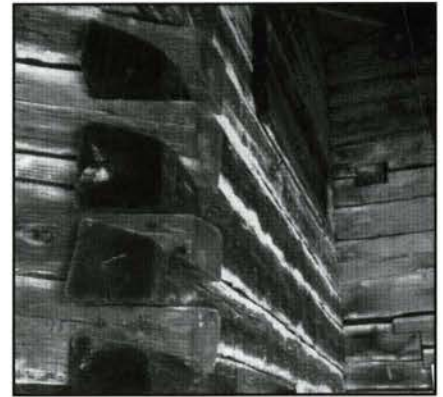
Fig. 17. An example of the dove-tailed joints and adzed half timber construction at Camp Harmony. (New Brunswick Museum, 1999)
