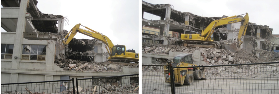
The manual demolition of the Chronicle Herald building in downtown Halifax, 2010; from "The Chronicle-Herald Building Is Being Destroyed," The Coast .
