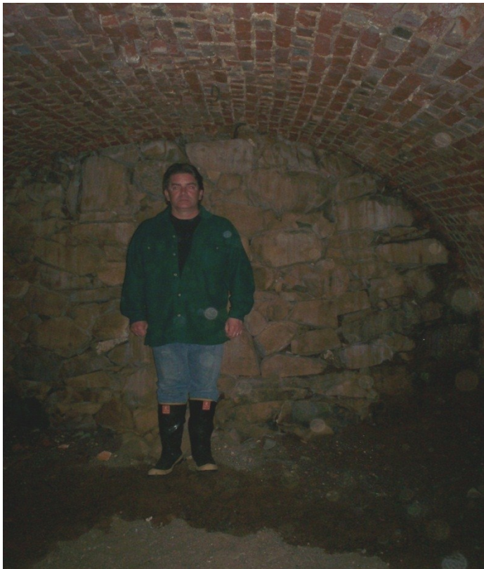
3.29 Image of the brick arch in the cellar of the Ruggles house. Note modern rock infill. (C. Cottreau-Robins, 2008)
